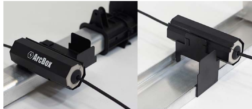
Installed with Flat Roof and Rack Mounted Solar
