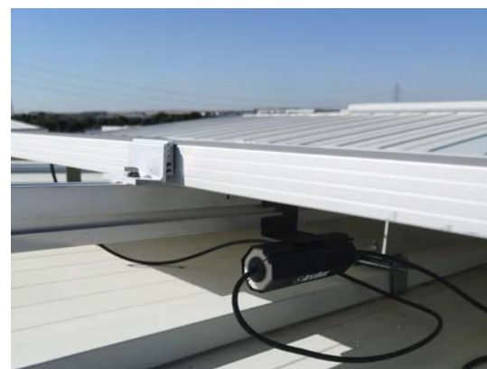
Madrid, Spain 100kWp for Industrial Building
