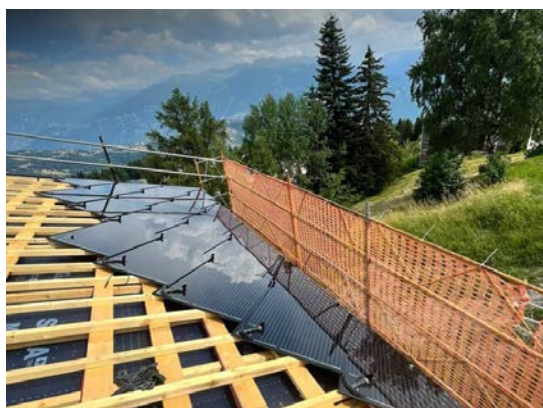
Sion, Switzerland BIPV tile system for mountain chalet
