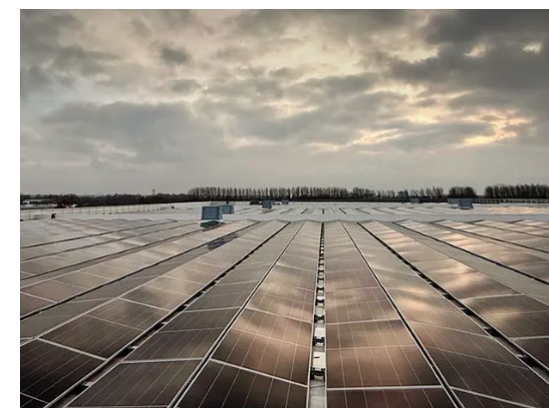
Oss, Netherlands 3.2MWp array for cold store warehouse
